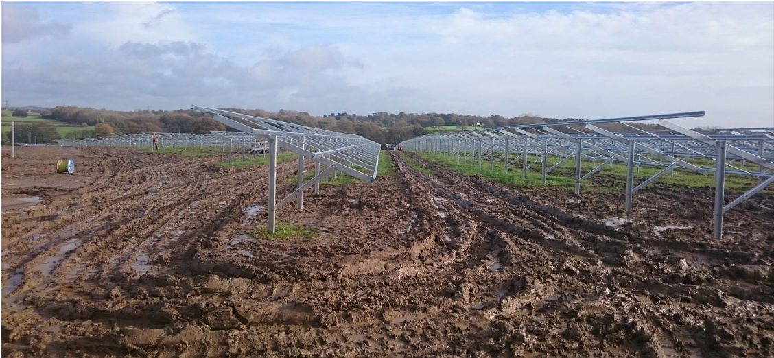
Inserts 36 and 37: Winter Installation (2015) and Operational Site (2022)
